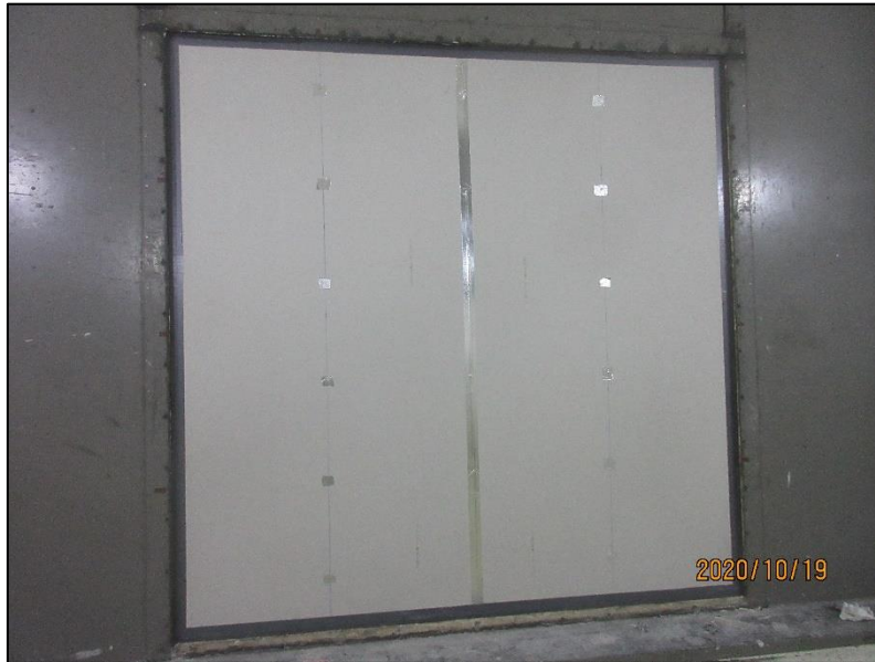
Photo No. 1 Receive Room View of Installed Specimen
